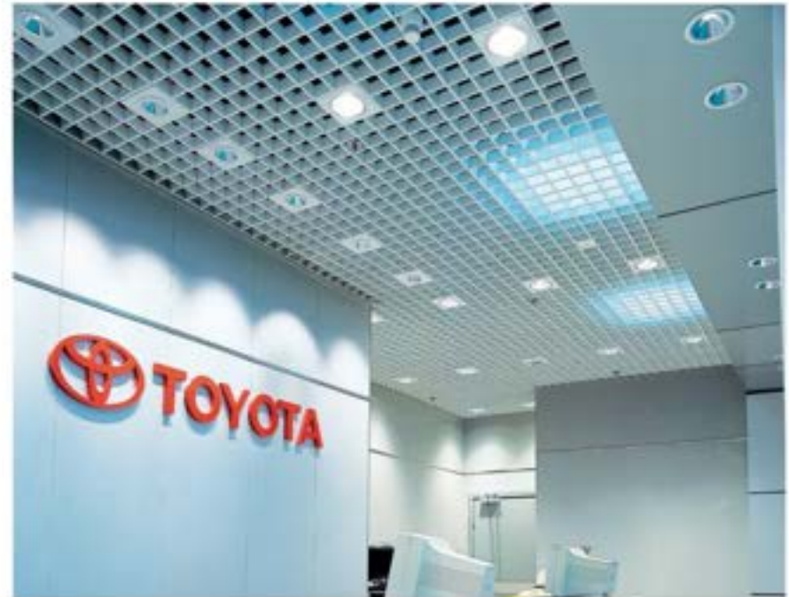
Ceiling system can integrate with lighting and other mechanical services
